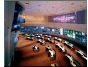
Network Operations Center
